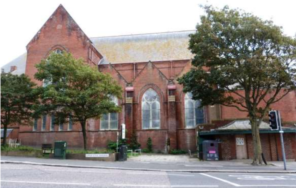
2. The Upper Rock Gardens elevation of St Mary's today - in urgent need of repair.
